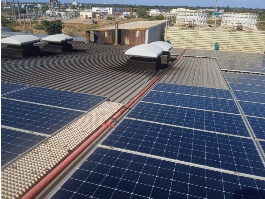
Figure 7: Solar panels exposed to an industrial environment on the roof of a factory (Midal Cables International)
