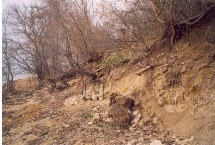
Fig. 2. General view of the destroyed river bank slope due to the impact of waves (photo of the authors)
