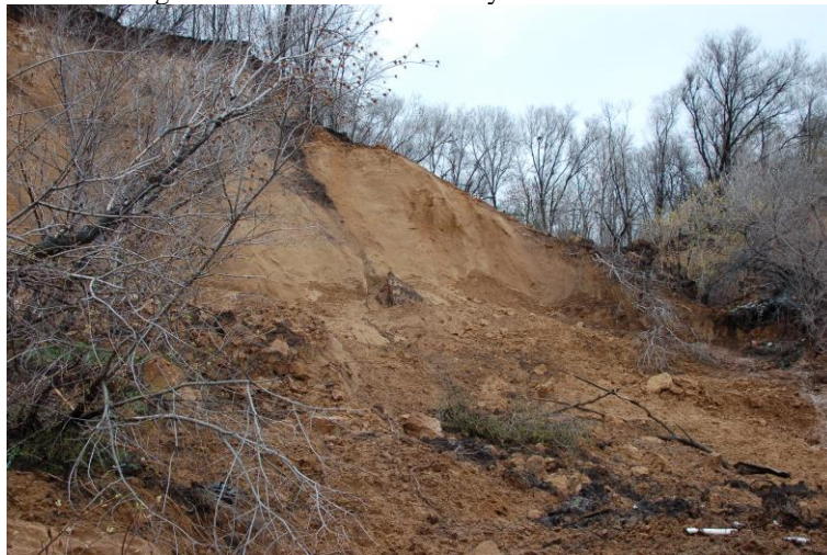
Fig. 3. General view of the destroyed riverbank slope due to the loss of stability (photo of the authors)
