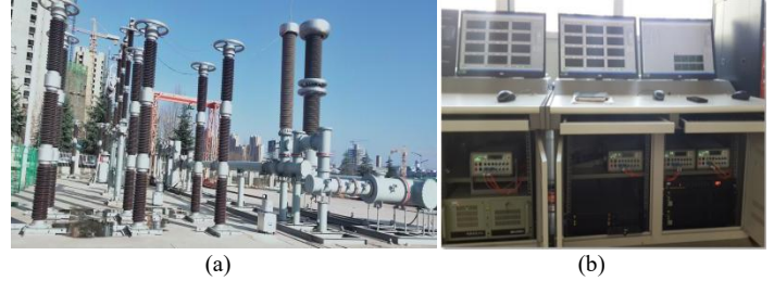
Fig.2. Outdoor experimental system structure (a) Outdoor test site of substation (b) System control room
