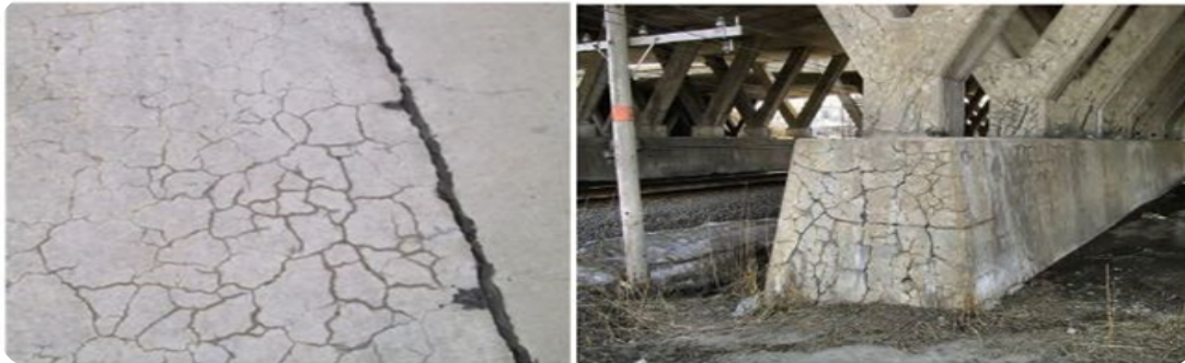
Figure 2. Infrastructure concrete cracking due to ASR
